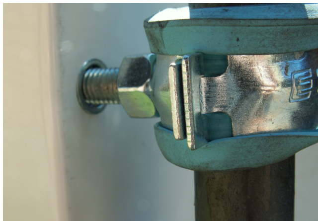
Close-up of attachment to cabinet.
