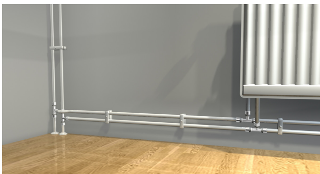
Example of clamping, visible installation
