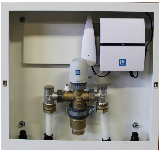
LK Mini Loop Valve M5 supplemented with LK ICS-RF1. The equipment is installed in LK Cabinet M5 WP-XL.
